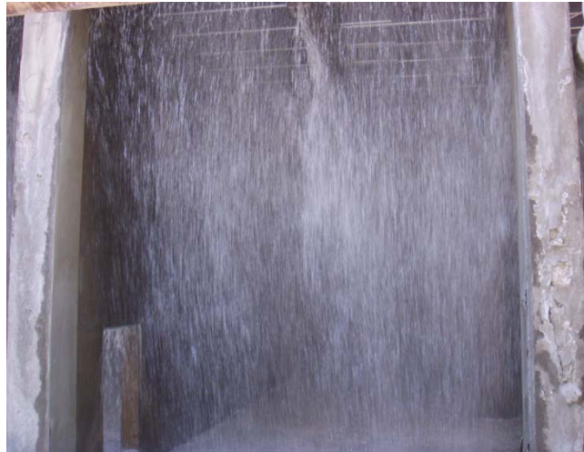
Figure 2b | Warm water spray inside the central plant cooling tower
